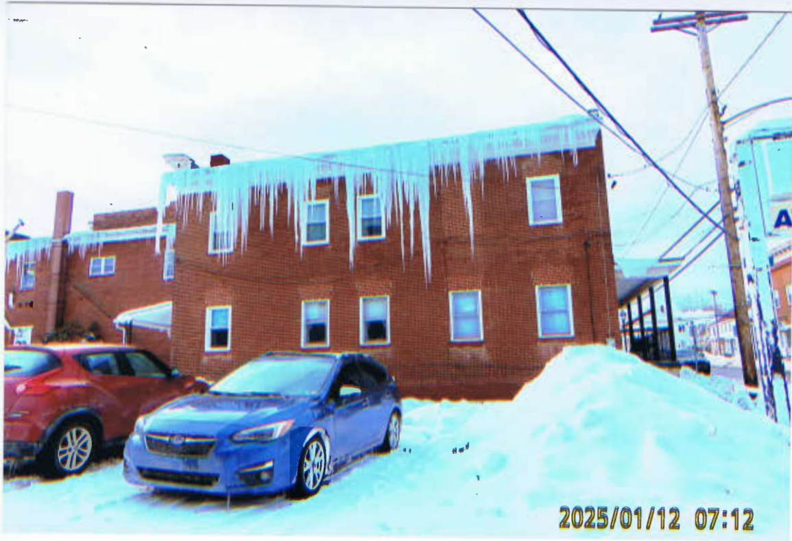
JANUARY'S ICE CYCLES HANGING ON THE ROOF OF LOIS HARRIS' HOME AS WELL AS LANDIS BAKERY. ADJOINING ALLEY CLOSED OFF FOR SAFETY PERPUSES.
